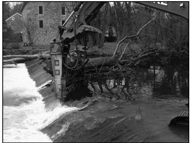
Removal of the Finesville Dam began on November 10, 2011. Gleim Environmental Group of Carlisle PA removed the dam using a design by Princeton Hydro engineers of Ringoes, NJ
