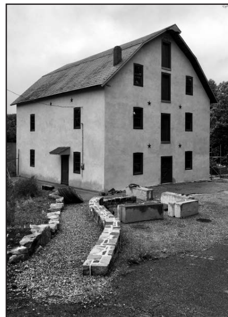
The scaffolding is down on the north wall of the mill, and the exterior restoration is really taking shape!!
